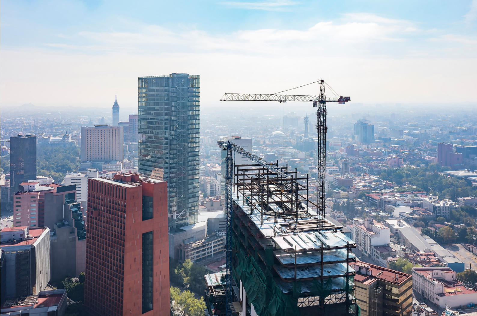
Aerial view of building under construction in Mexico City, Mexico. Credit: Erich Sacco/Adobe Stock
