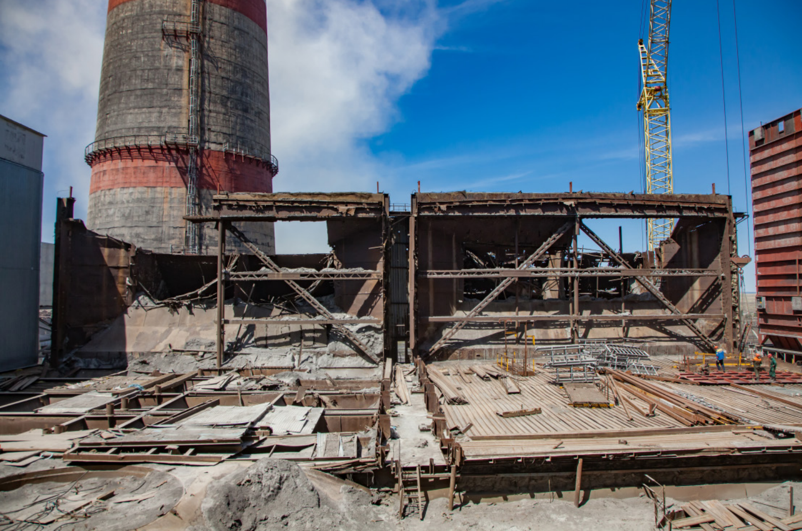
Demolition of coal bunkers at the GRES-1 power station, Kazakhstan. Credit: Alexey Rezykh/Adobe Stock
