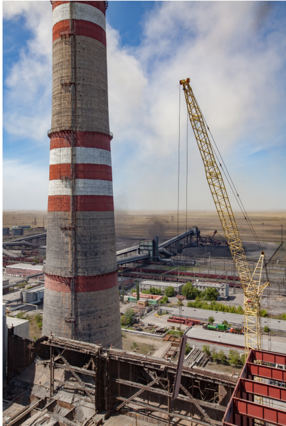
Demolition of coal bunkers at the GRES-1 power station, Kazakhstan. Credit: Alexey Rezykh/Adobe Stock
